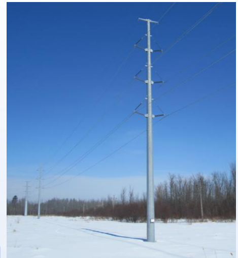
The new Amber – Donaldson Creek poles are similar to the one shown here.
